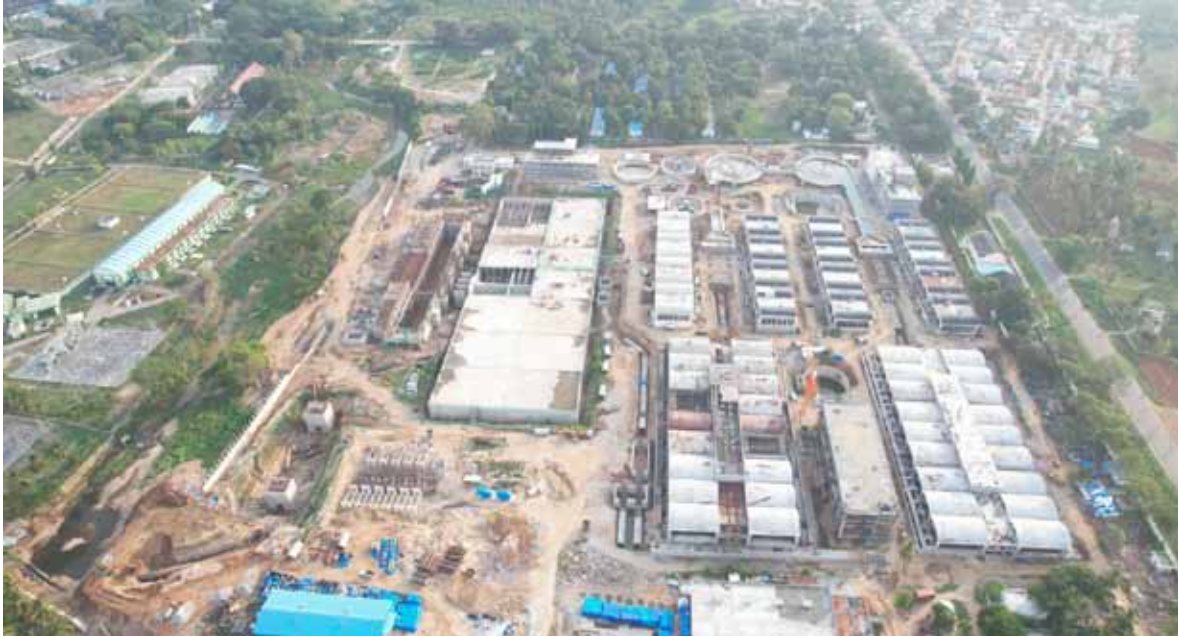
Kaveri Water Supply 5 th Stage - Water Treatment Plant and Pumping Station at T K Halli under construction
