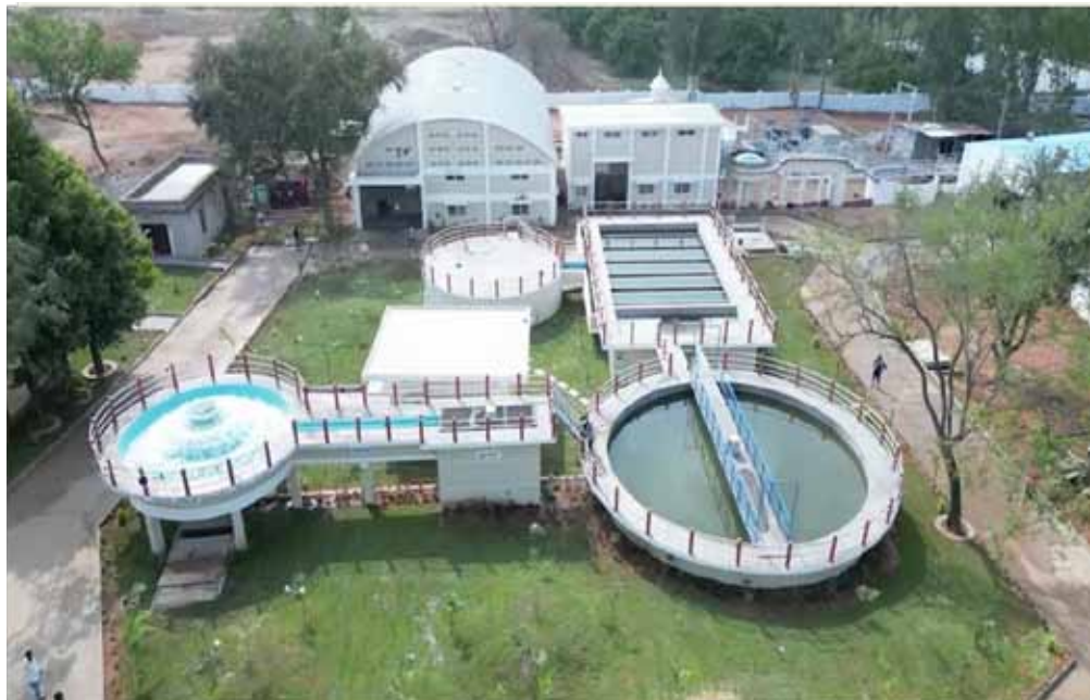
13MLD Capacity WTP under 2 nd Stage WSS to Shorapur & 3 Enroute Villages with Krishna River as Source
